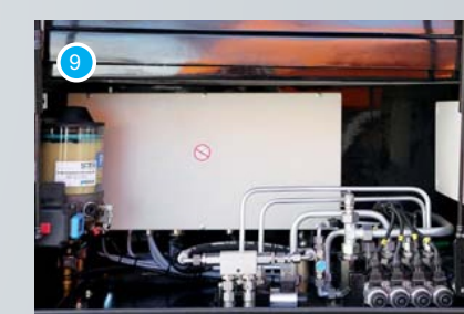
The efficiently arranged control centre
